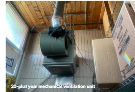
20-plus year mechanical ventilation unit
